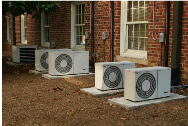
Air Source Heat Pumps
