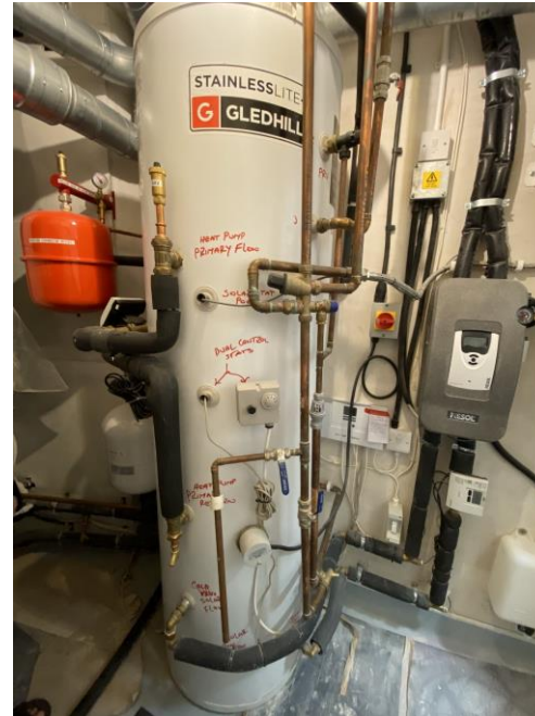
Water Tank System
