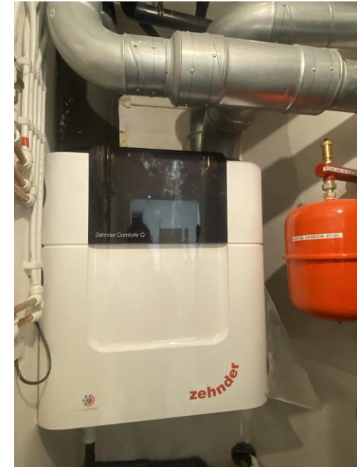
Air Source Heat Pump System
